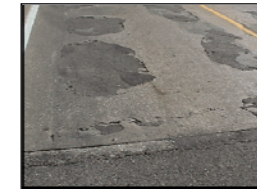
Delamination w/ patching
