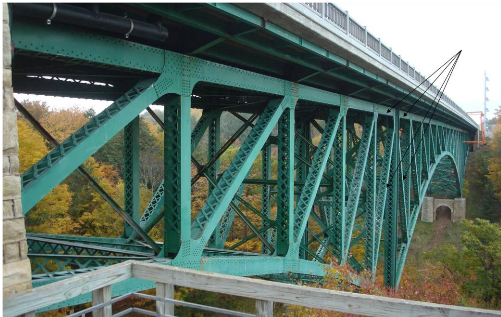
Figure 1: Location of Sensors on Cut River Bridge
