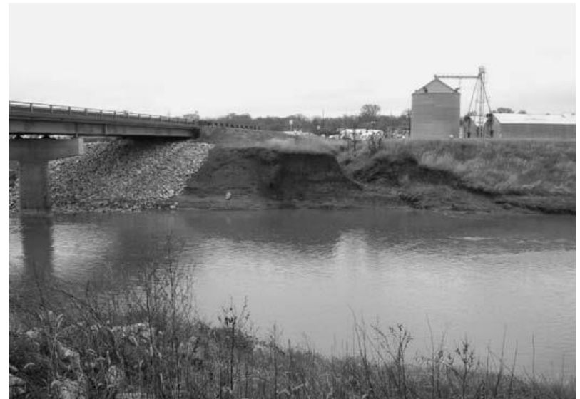
Erosion due to surface runoff threatens roadway
