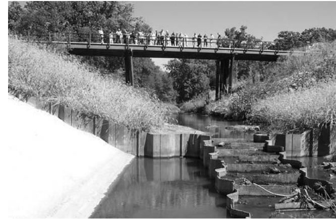
Sheet pile weir (with fish ladder)
