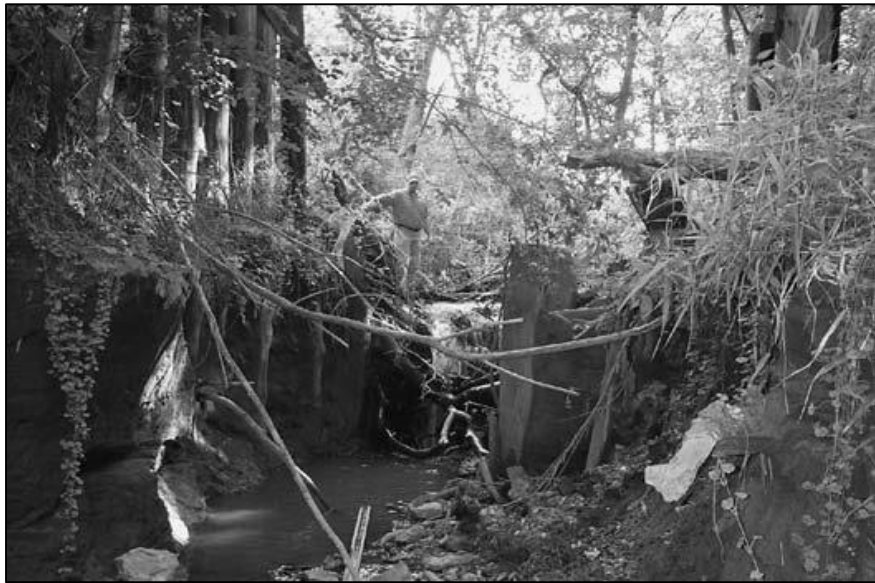
Upstream progression of head cut through waterway exposes pier supports and destabilizes abutments
