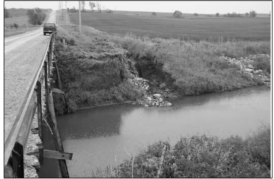
Erosion of side drainage in embankment close to abutment exposes it to scour
