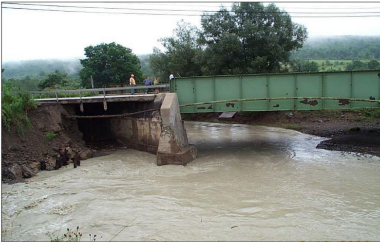
Bridge abutment critically compromised by scour 1
