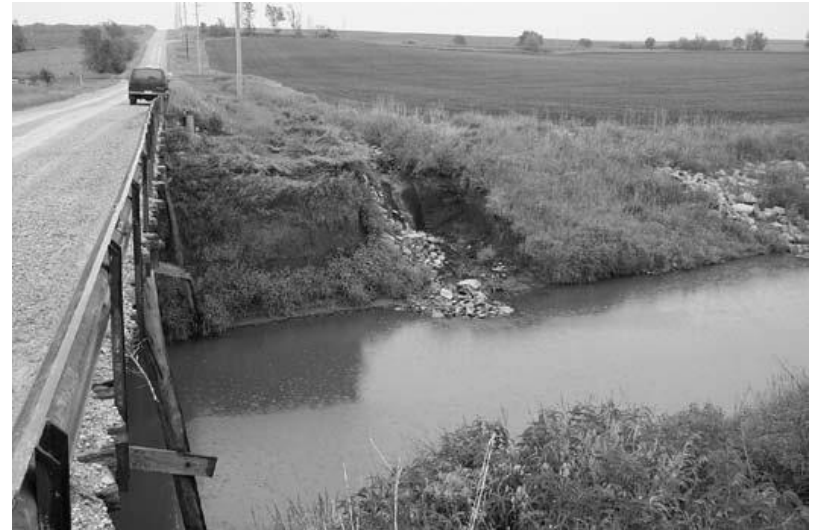
Erosion due to surface runoff increases scour exposure
