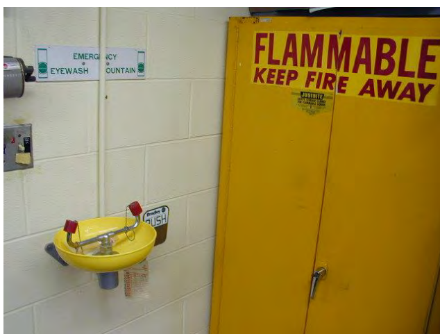
Figure 6.1 – Flammable Storage Cabinet
