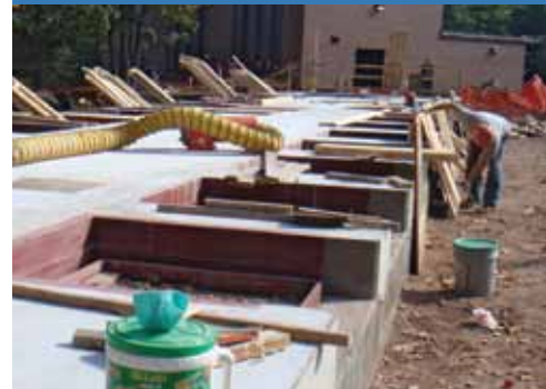
Adjunct Professor Erik Lilleskov observes the construction progress at the mesocosm site.
